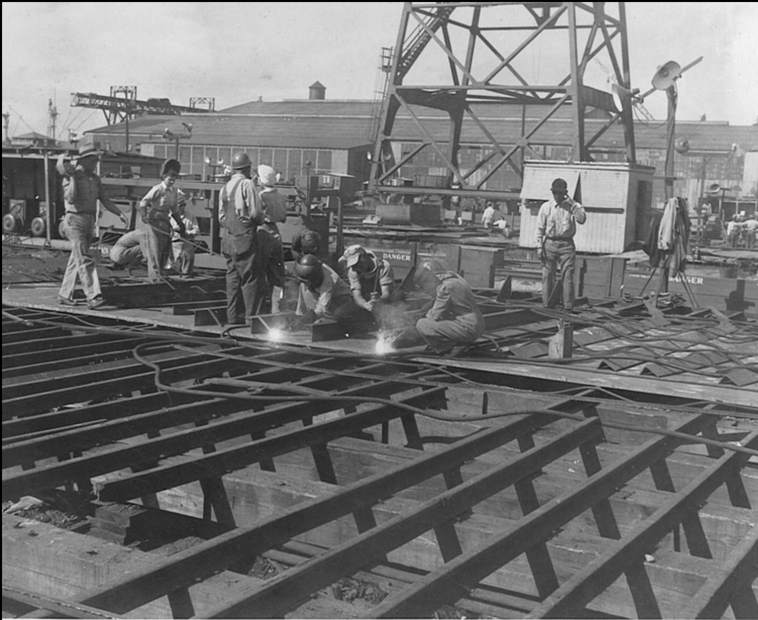
Welding instead of rivets (jaj146)
